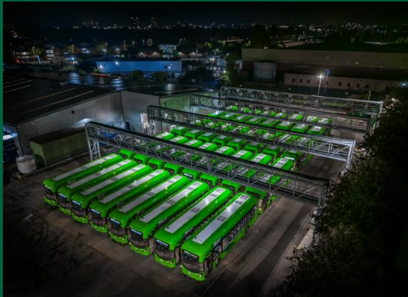
Figure 11: Overhead charging gantries at First Bus's depot in Leicester.
