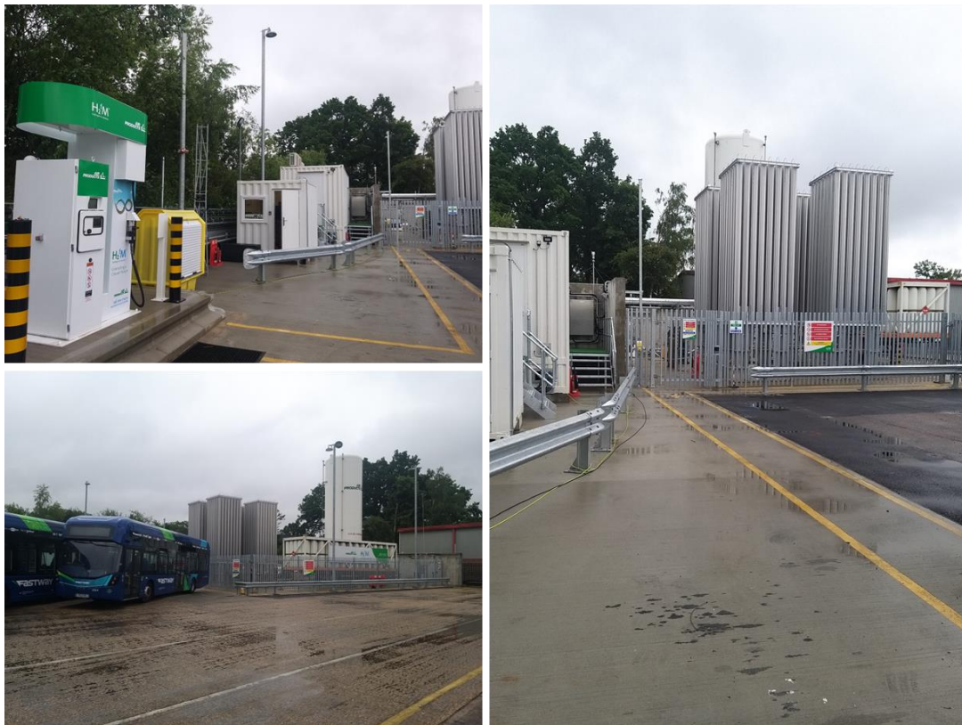
Figure 13: View of the HRS secure compound; vaporiser in the foreground (right picture) – LH2 tank (tall white structure), with a gaseous hydrogen tube trailer in front (lower left picture) – dispenser unit (upper left picture)
