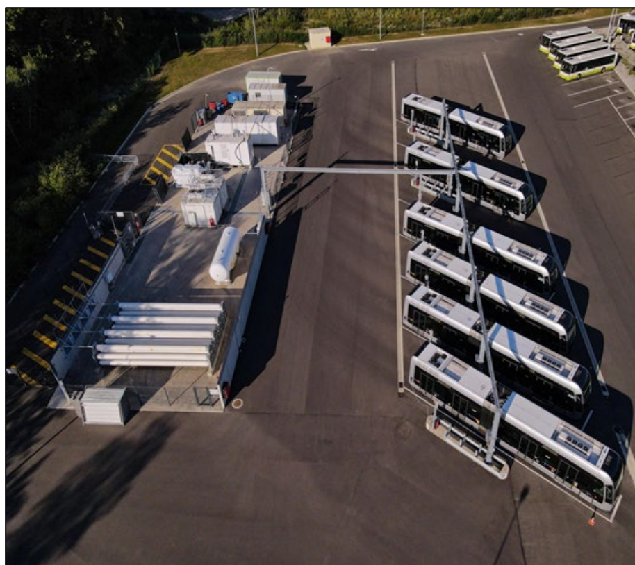
Figure 4-4: HRS with on-site hydrogen generation in Pau, France.
